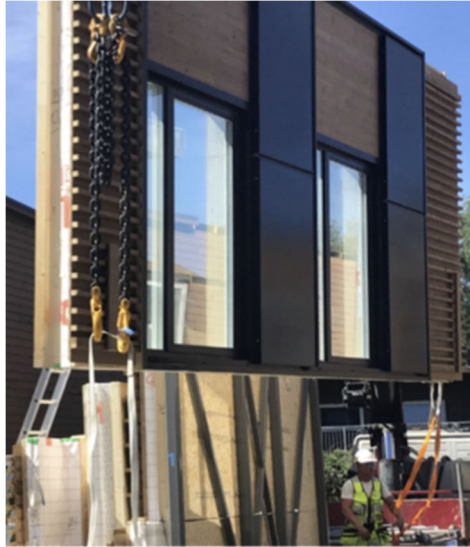
Figure 59. Prefabricated facade elements with PV panels being installed during a deep retrofit.
